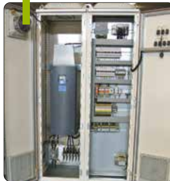
Winch control cabinet with frequency converter
