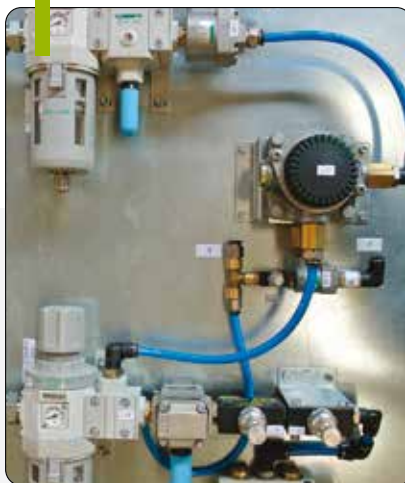
Winch pneumatic control panel
